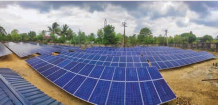
250kWp Solar power plant at 66kV KSEB Substation Kozhinjampara, Palakkad
