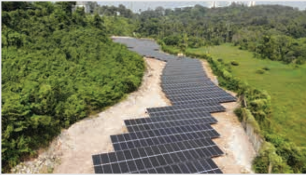
2.25 MWp Solar power plant at KSEB BDPP - Brahmapuram
